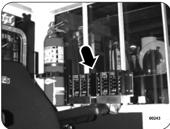
Figure 7: Control Boxes For The VOAC Control Valve
