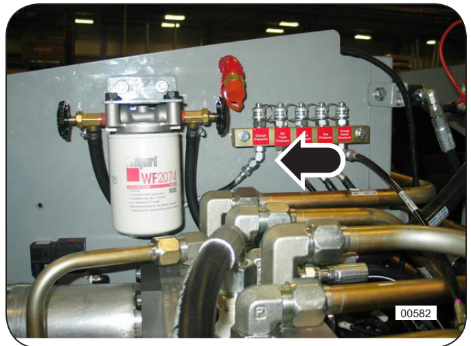
Figure 11: Drive Pump Pressure Gauge Port Tap
