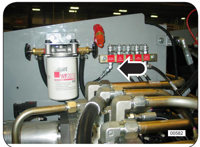
Figure 8: Drive Pump Pressure Gauge Port Tap
