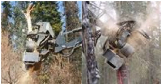
A rubber-tired 630 TimberPro carrier equipped with a Rolly chipper gives Alberta’s Triple G Construction the mobility and productivity it needs to tackle mountain pine beetle control contract work.
